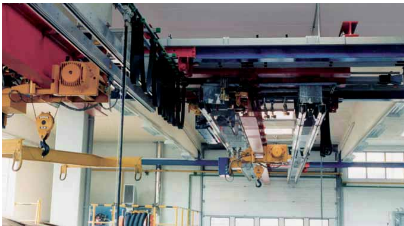
Aluminium enclosed conductor system on crane bridge.
