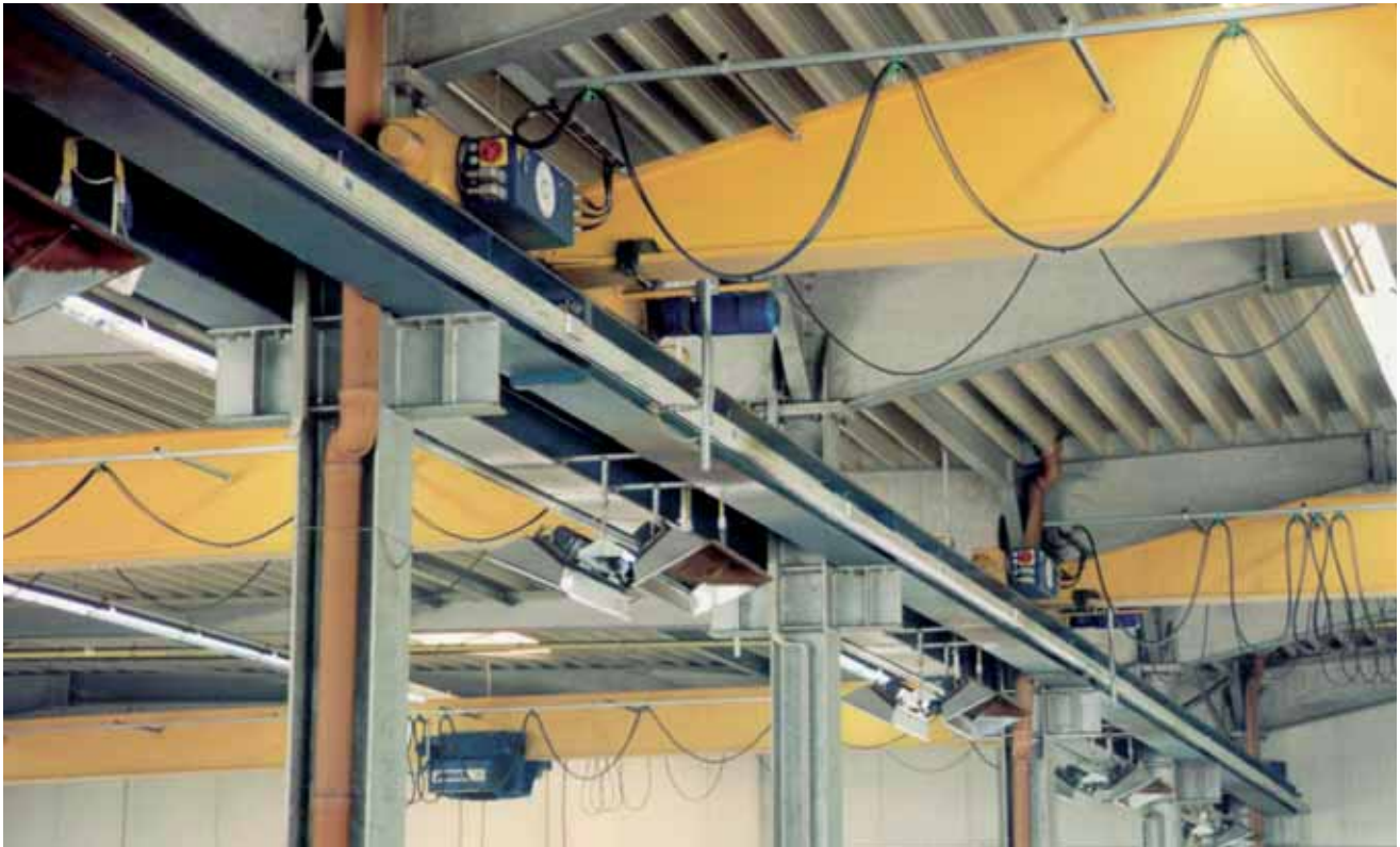
Aluminium enclosed conductor system for crane electrifications.
